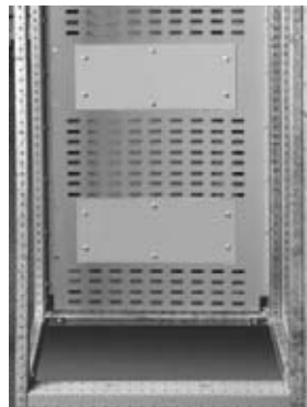
Rear cable area.
